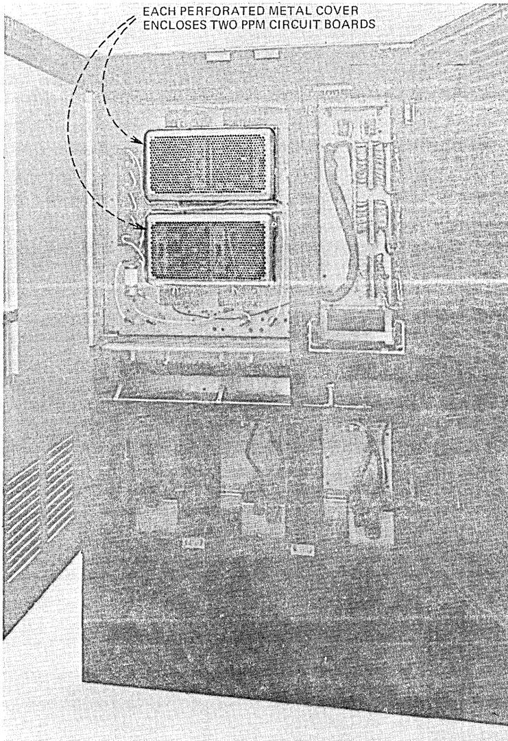
Fig. 7—Pulse-position-modulators shown in the high-voltage area of a converter bay.
