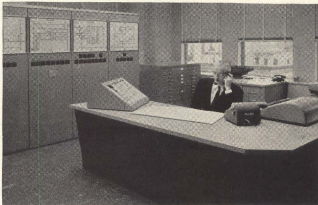
Automatic data acquisition and display gives true "fingertip" control to dispatcher J. H. Philips, enabling him to distribute peak day-loads up to 750 million cubic feet of gas to Peoples' 275,000 customers.
