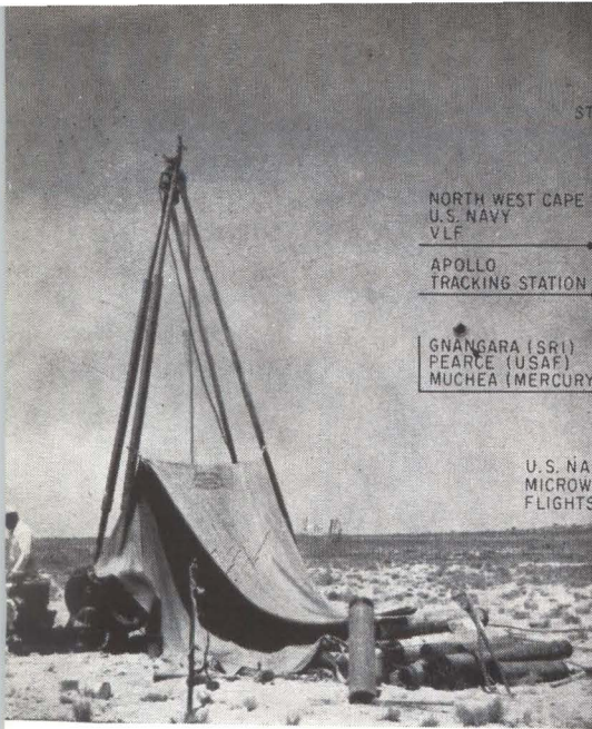
DRILLING RIG probes shimmering white limestone salt flat, to insure there will be no caverns under tower foundations at Navy's vlf station
