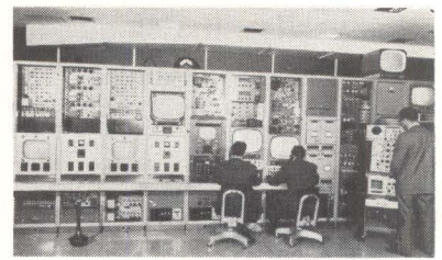
PENTAGON SYSTEM can distribute four different programs simultaneously to different viewing areas
