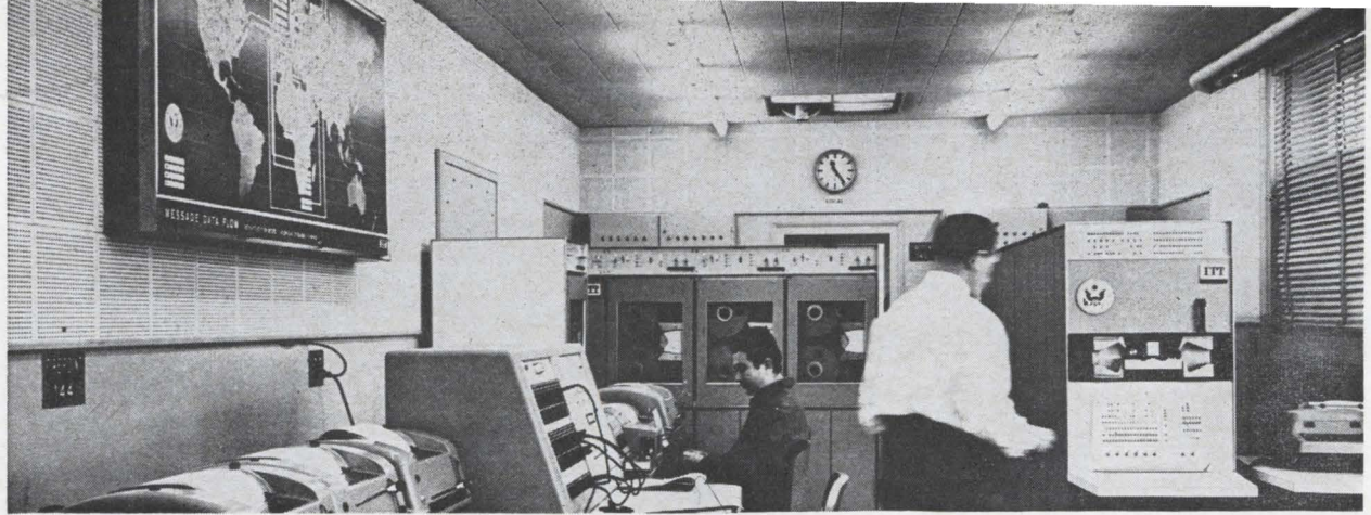
Nerve center for the State Department's communications operations in Europe is this Paris facility that switches and processes digital information. Developed by International Telephone and Telegraph Corp., the system accepts information from high-speed computers and slow-speed teleprinters, and stores low-priority messages for later transmission.
