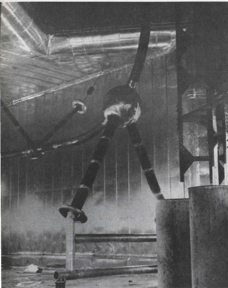
Anticorona fittings applied to the high-voltage trunk at Navy radio station in Cutler, Me. The room is copper-shielded to prevent eddy currents in building structure.
