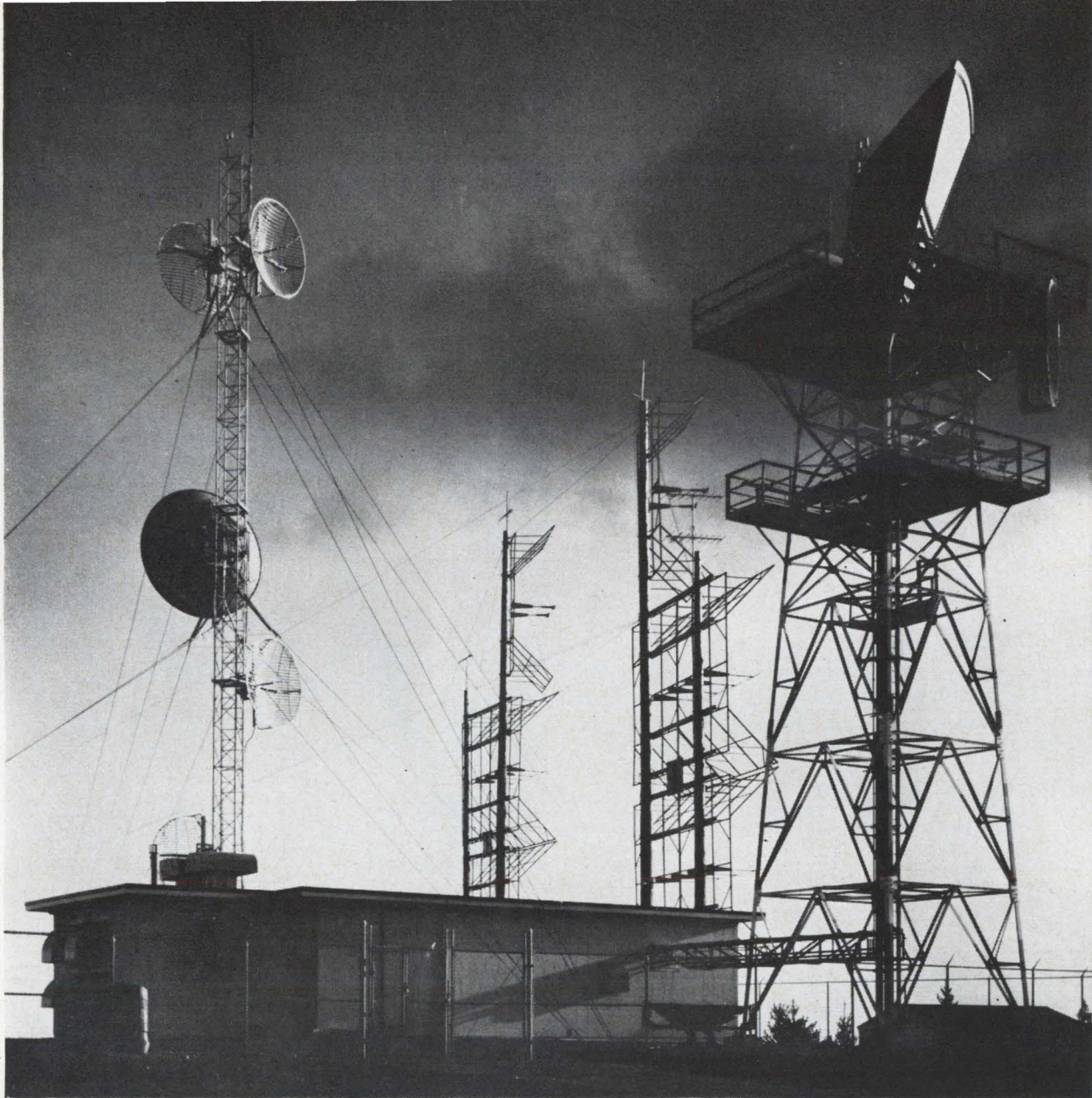
Microwave repeater system for television transmission, similar to the system shown operating in Canada, will be supplied to Yugoslavia by the General Telephone & Electronics Corp.'s Italian subsidiary, Marelli Lenkurt S.p.A. The equipment, costing $1 million, will consist of four microwave links operating over 600 miles.
