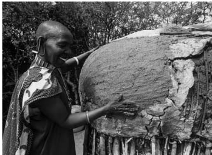
A builder uses a traditional plaster mix incorporating cow dung to maintain her house. Photo: Practical Action / Neil Cooper.
