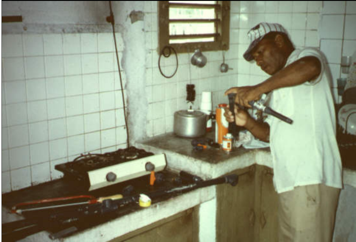
Final touches on a piping system with PVC pipes Photo: Krmer (TBW)
