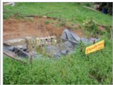
Fig 1: Marsh before renovation
