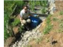
Fig 12g: Adding rocks to highlight the piping layout on surface of soil. This adds an artistic element to the system and allows for easy location of the system for
