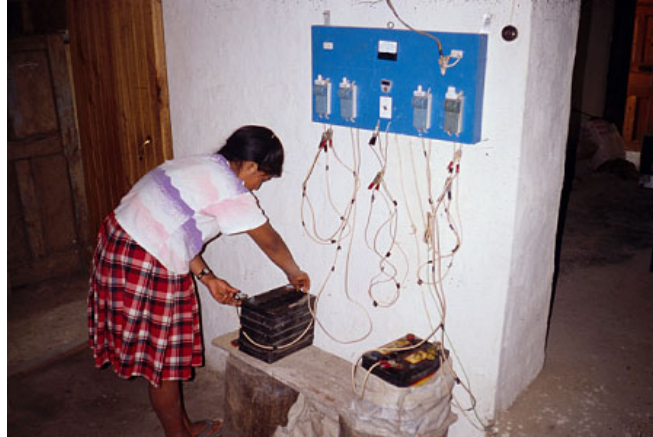
Figure 2: Nilde Portal charging the batteries. Her family owns an improved mill at Cuichupucro to which local villagers bring their grain. Photo credit: Practical Action / Steve Fisher
