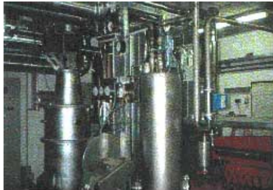
Wood gasifier for co-gen set
