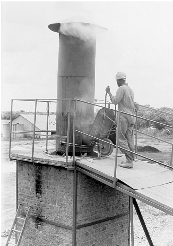
Figure 1: Loading stone/fuel through the hopper at the chimney level, lime kiln, Chegutu, Zimbabwe Photo: Practical Action / Kelvin Mason.
