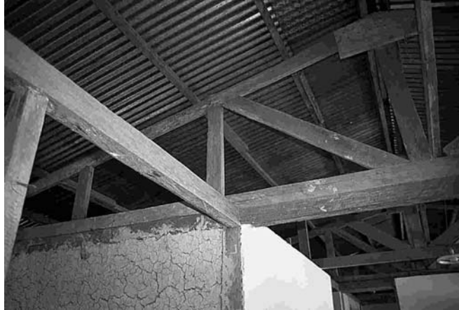
Figure 9: Careful jointing between columns and beams improves structural integrity ©Practical Action /Chris Martin
