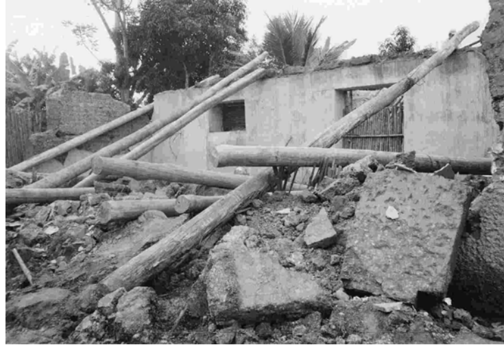
Figure 2: The impact of the earthquake on a tapial house in Soritor © Practical Action/Megan Lloyd-Laney
