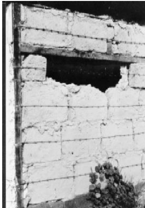
8-5 Dangerous solution, Chile
