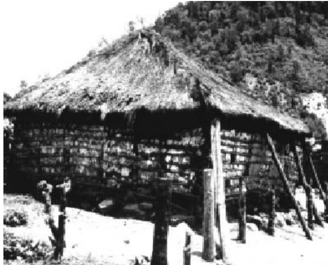
5-2 Wattle and daub structure, after a heavy earthquake in Guatemala (Minke 2000)
