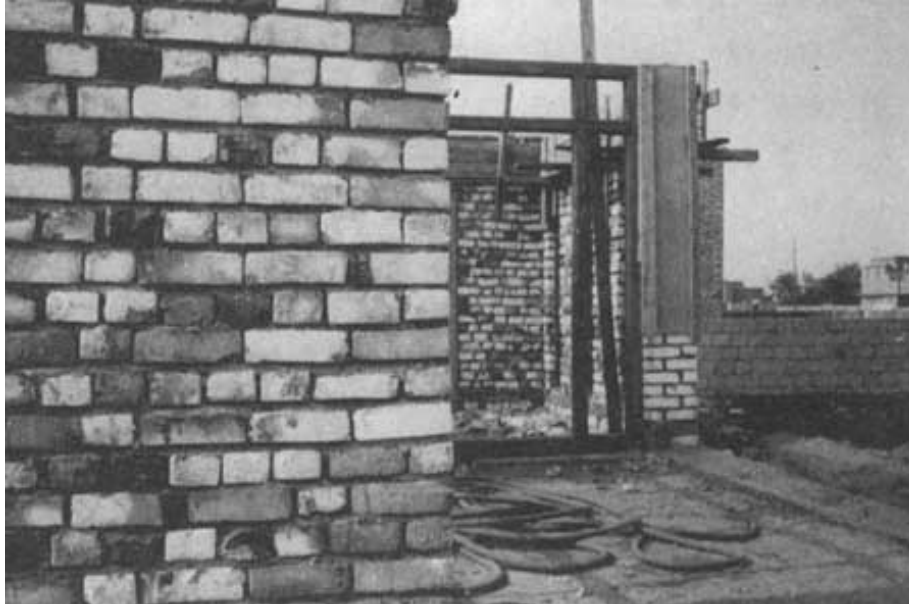
Figure IV.3 - White efflorescence on brickwork (Middle East)
