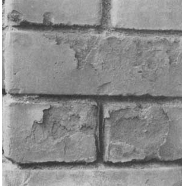
Figure IV.4 - Flaking of the type produced by soluble salts (India)
