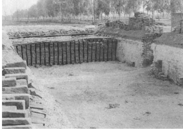
Figure VII.20 - Cross-link bricks between the separate bungs or pillars of bricks in Bull's Trench kiln
