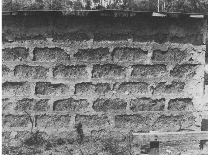
Figure I.1. Unstabilised soil blocks after 3 year's exposure in Ghana
