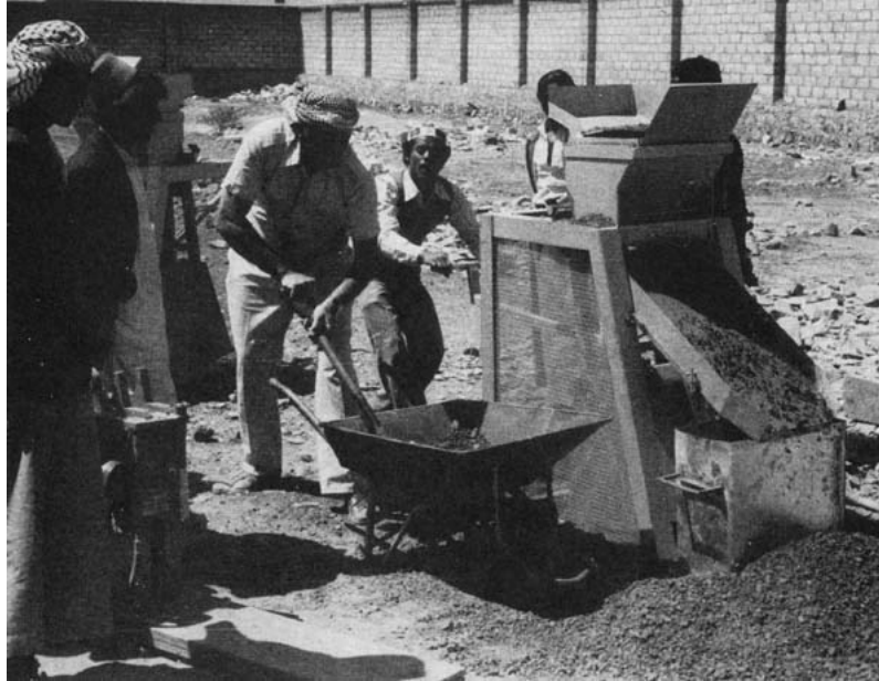
Figure III.3. One-man pendulum crusher in operation
