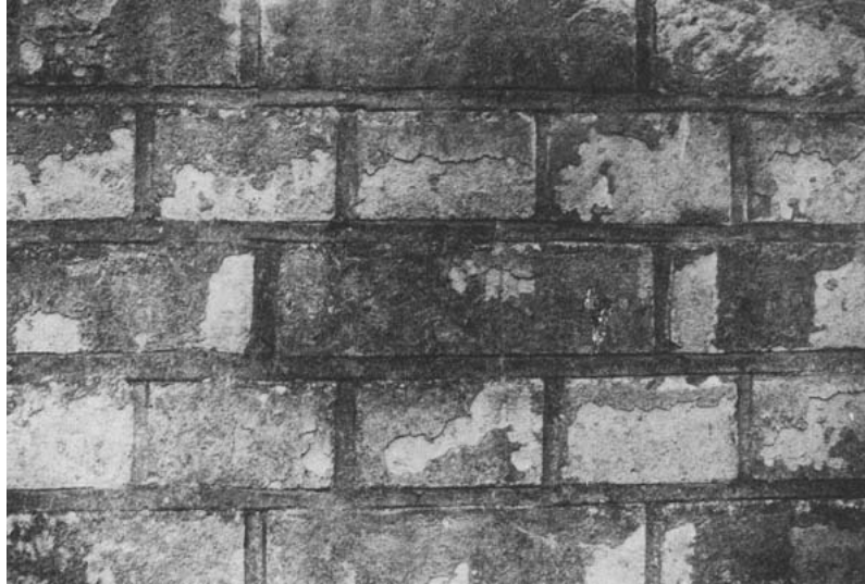
Figure I.3. Wall made of cement-stabilised soil blocks after 33 year's exposure in the United Kingdom
