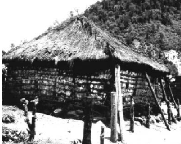
5-2 Wattle and daub structure, after a heavy earthquake in Guatemala (Minke 2000)
