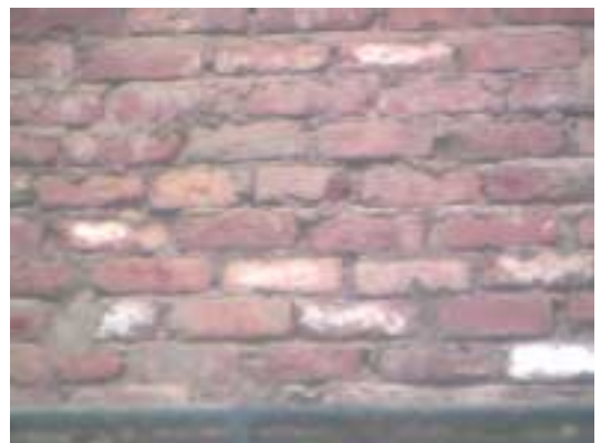
Poorly fired bricks
