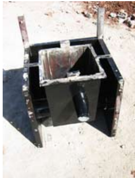
Formwork for the manhole, viewed from the side of intake (front panel removed)
