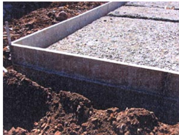
A formwork for foundation, panels mounted on top of each other, side by side and at the edge
