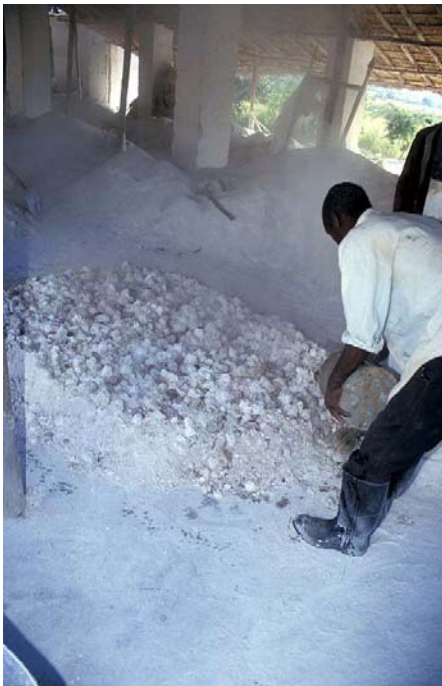
Figure 3: Hydrating of quicklime using a watering can Chenkumbi Limeworks, Malawi © Practical Action/Dave Mather
