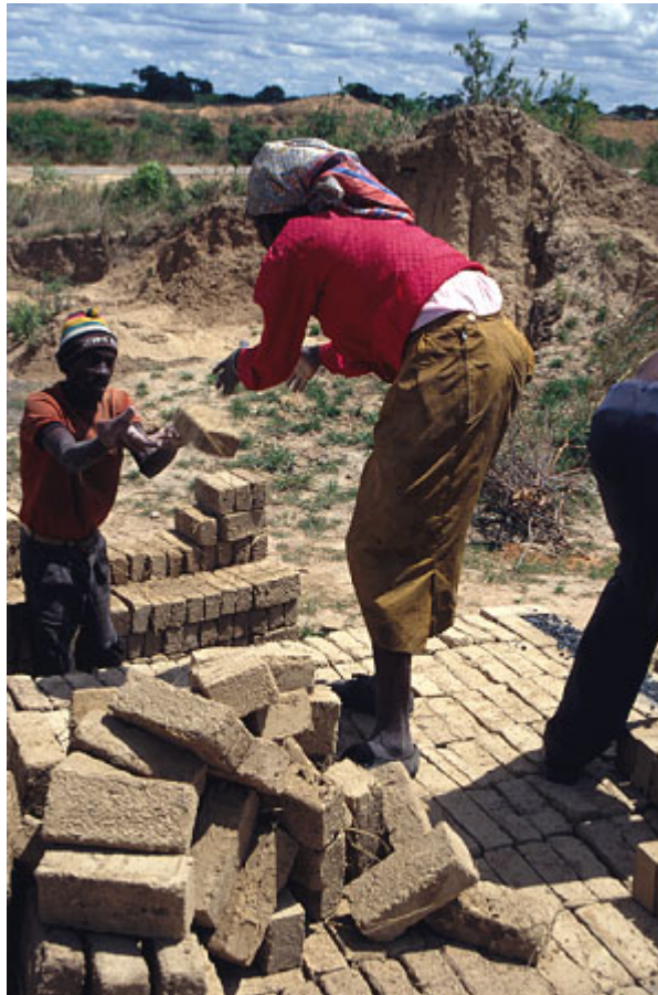
Figure 2: Brick makers are shown building the clamp kiln prior to firing, Zimbabwe ©Practical Action/ Janet Boston
