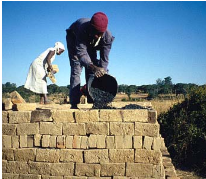
Figure 1: Boiler waste is sieved and used as a fuel for firing brick clamp kilns at Kurewasekwa Cooperative in Epworth, Harare ©Practical Action / T. Schilderman
