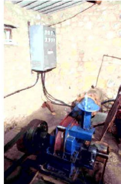
Nyafaru, Zimbabwe, inside the power house
