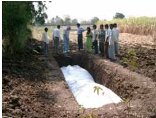
A newly installed 10,000-liter storage unit installed in a 1-meter wide by 1-meter deep by 10-meter long trench.
