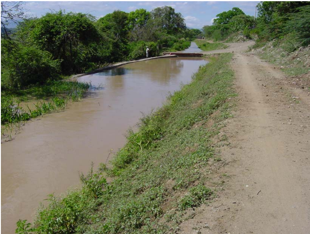
A canal with impending spillage (zero freeboard).
