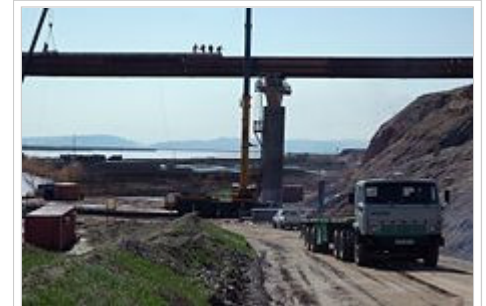
Construction of the Afghanistan-Tajikistan Bridge which was completed in August 2007 and is now the largest bridge in Central Asia.
