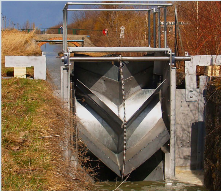
Fig.1: Stem Pressure Machine, downstream view of pilot plant
