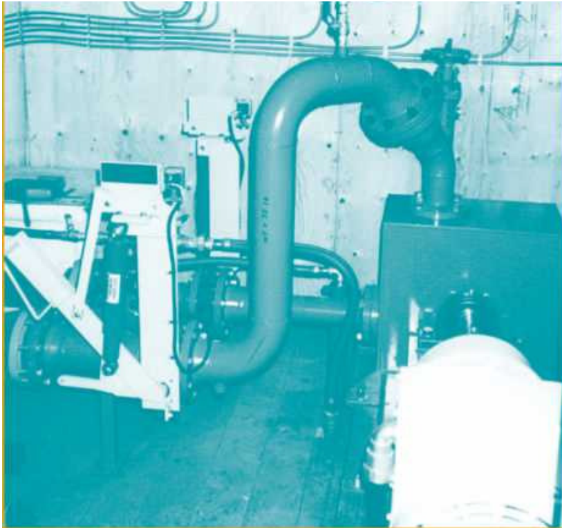
Figure 30. Equipment inside a powerhouse (photo courtesy of Thomson and Howe Energy Systems Inc.)
