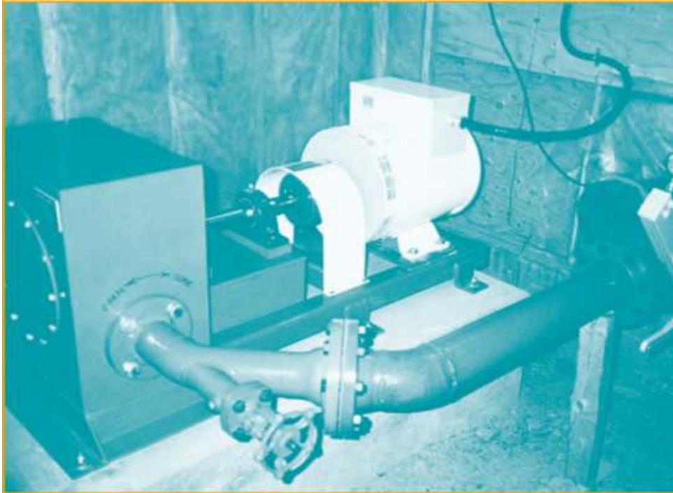
Figure 19. A directly coupled Pelton turbine with synchronous generator 8-kW system
