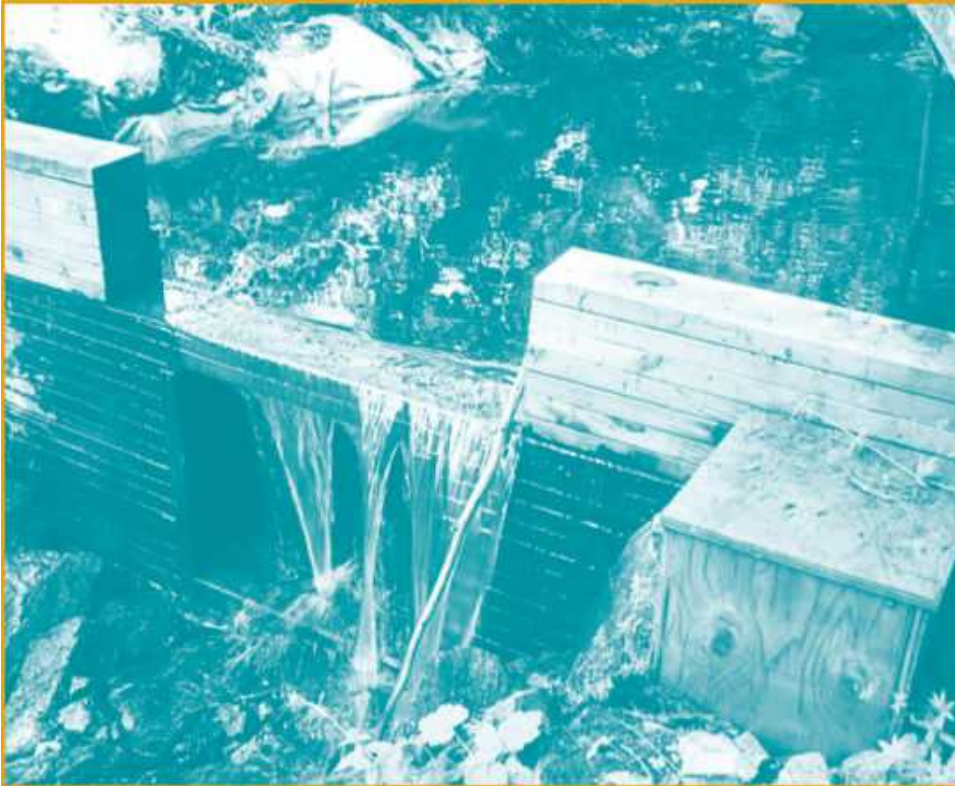
Figure 12. Intake for a 2-kW micro-hydropower system (photo courtesy of Homestead Hydro Systems)
