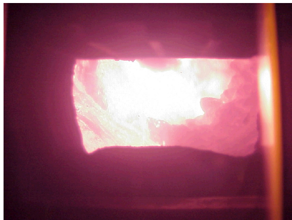
Figure 4.11: Interior view of an operational wet kiln (Copyright Halliburton Energy Services).
