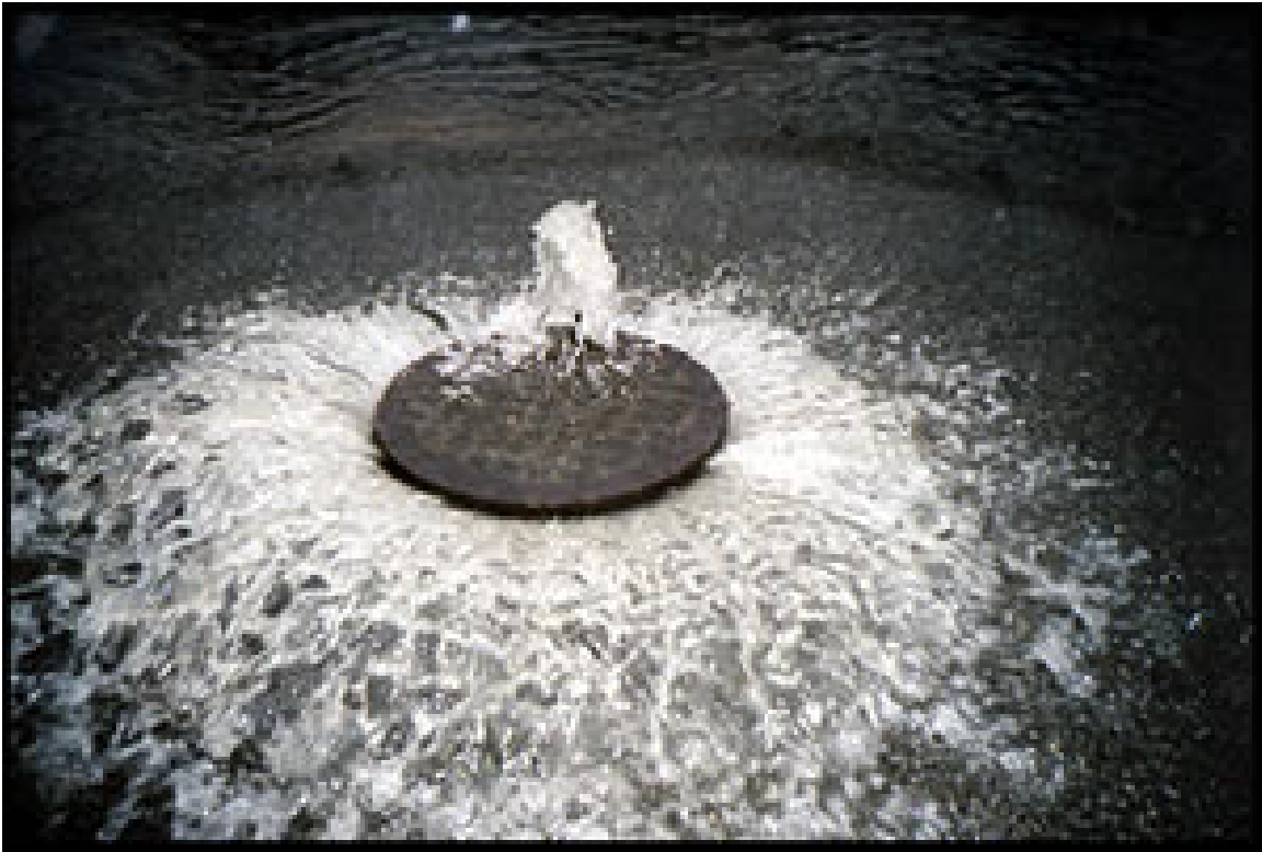
Figure 5.40: Overflowing Sanitary Sewer A manhole cover blown off by a June 2006 sanitary sewer overflow in Rhode Island. Source: U.S. Environmental Protection Agency 47 via Wikimedia Commons
