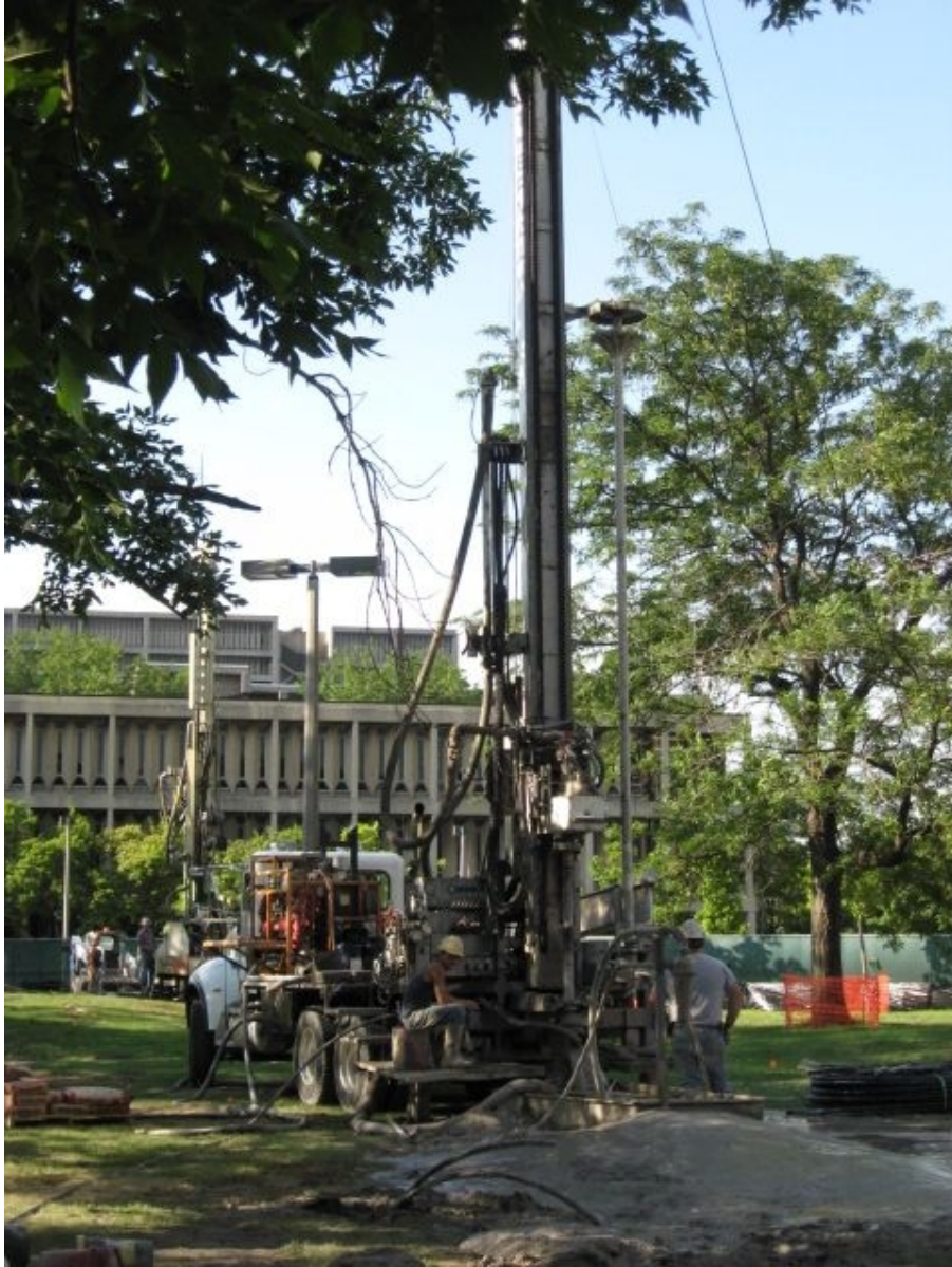
Figure 8.15: Installing a Geothermal Pipe System Drilling to install geothermal ground source pipe system. Source: Office of Sustainability, UIC 46
