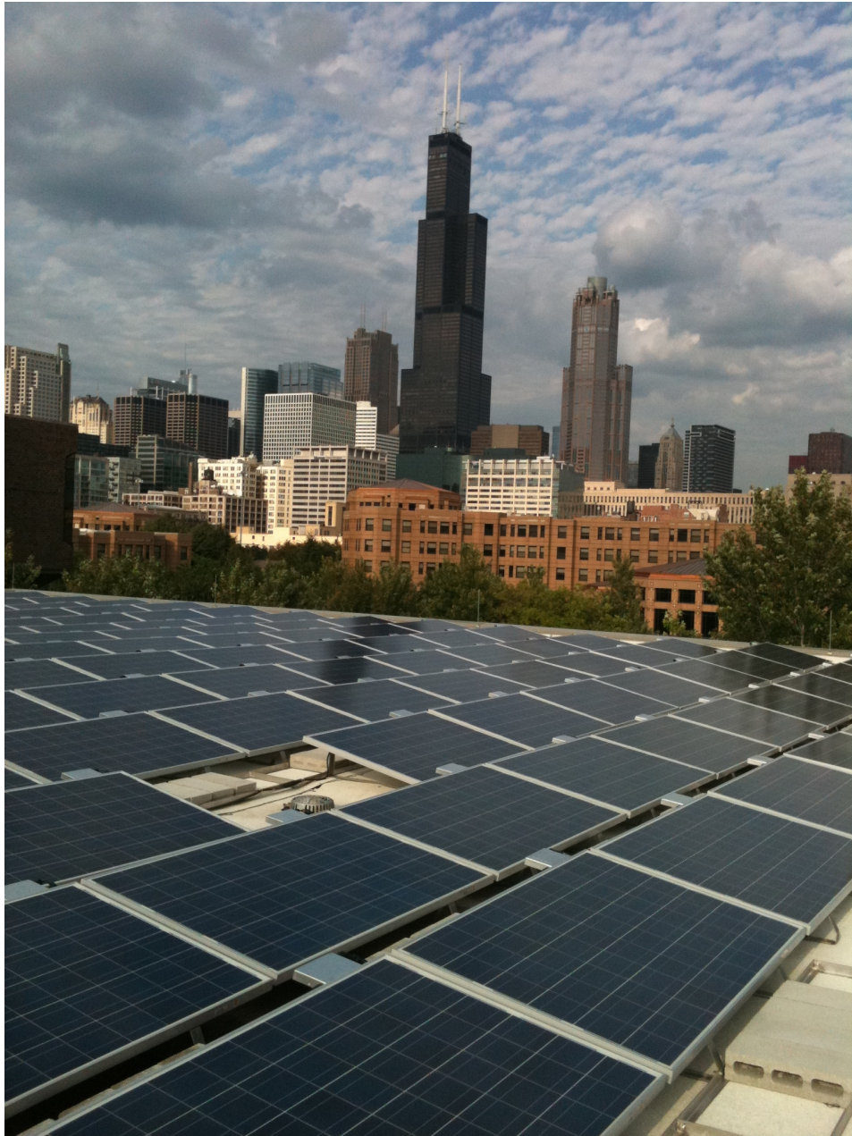
Figure 8.16: Rooftop Solar Installations Rooftop solar installation on Douglas Hall at the University of Illinois at Chicago has no effect on land resources, while producing electricity with zero emissions. Source: Office of Sustainability, UIC 48
