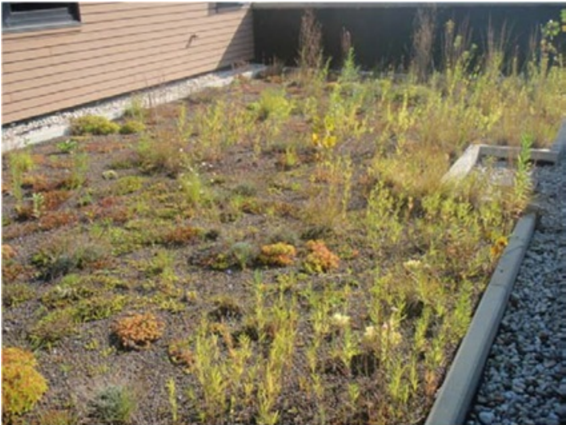
Figure 11.8: A Green Roof The green roof on this police station in Village of Villa Park, Illinois has shallow-rooted plants placed in a thin layer of growing medium installed on top of a waterproof roof membrane. Source: Jaffe, M. et al. (2010) (p. 542), Fig. 13, p. 116.
