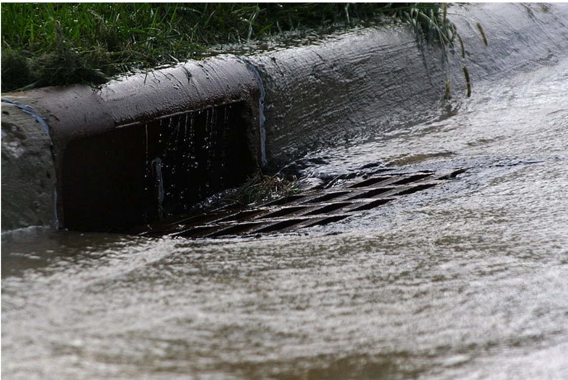
Figure 5.46: Storm Drain Curbside storm drain receiving urban runoff. Source: By Robert Lawton 53 via Wikimedia Commons
