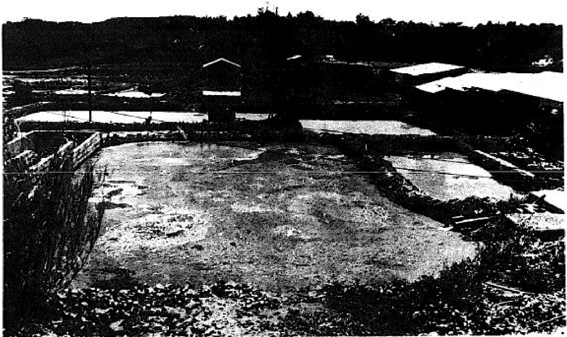
121890_illustration 2-12_Sludge Conditioning Plant page 121890_125b of 248
