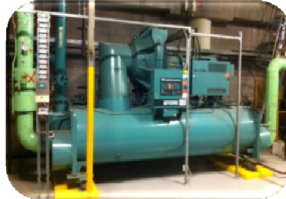
27 air conditioning Water Chillers
