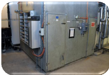
2900 Air conditioning units
