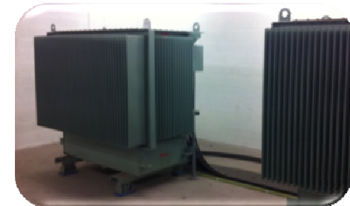
35 high voltage substations
