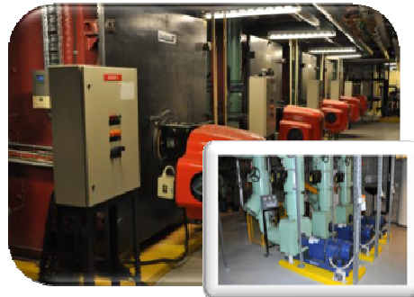
229 air-conditioning pumps & 31 Boilers
