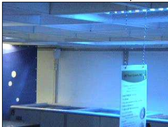
The technical zone: the CRACs
