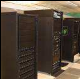
smarter data center
