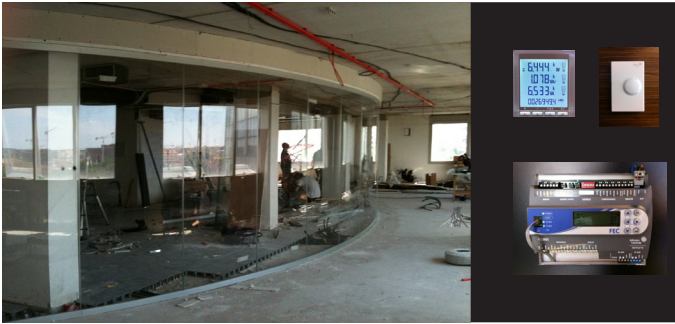
Figure 2: Integration of sensors and meters during renovation
