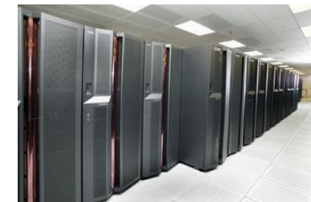
Technology Assets in a Green Data center reporting heat and energy issues
