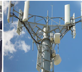
Infrastructure: Telco, Utilities
