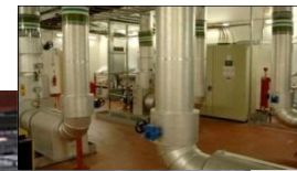
Fully resilient air conditioning
