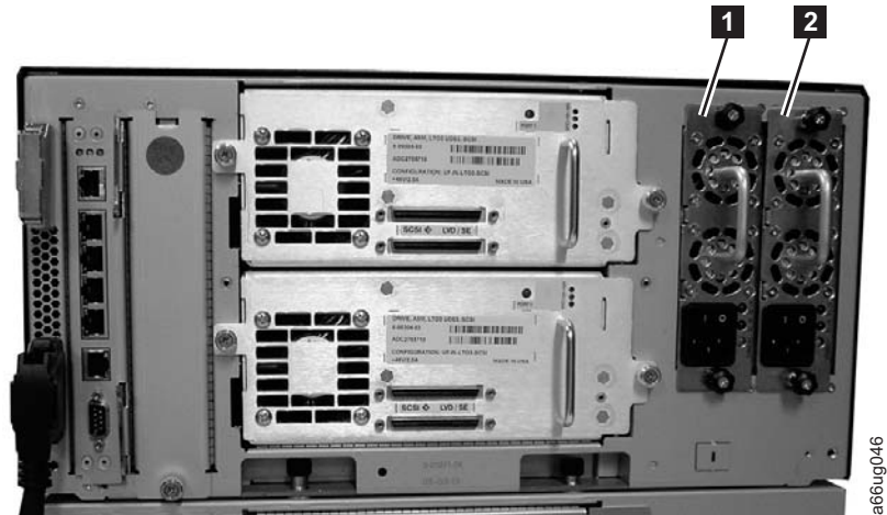
Figure 12-19. Power supplies in a control module
