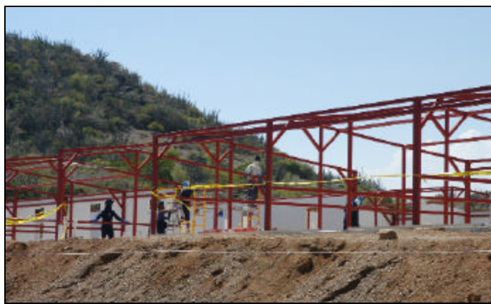
Photo by Spc. Katherine L. Collins Construction workers assemble the framing for various structures within Camp America North North.
