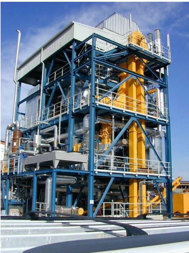
Fig. 18. Biomass CHP Plant
