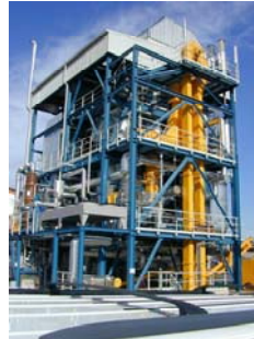
Biomass CHP Plant
