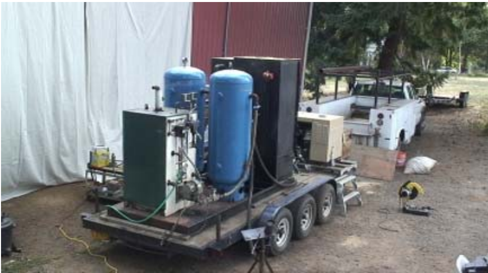
Fig. 17. Crorey Biomass Gasifier
