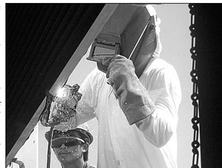
Kvaerner welder Angelo Esquerra fixes a garage door on the HAZMAT building while fellow crew member Ramil Magtoto assists.
