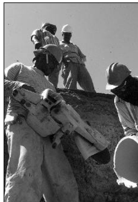
Workers with Radcliffe Construction Inc., Kvaerner's main subcontractor, trim a new water pipe for installation in a joint project along Sherman Avenue.
