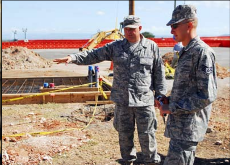
Air Force Master Sgt. Daryl E. Smith Jr. gives direction to Air Force Staff Sgt. Guy Conley while working on the Shore Power project. When the project is completed, Camp Justice will be supported by the commercial power on base instead of generator power. – JTF Guantanamo photo by Army Sgt. Michael Baltz
