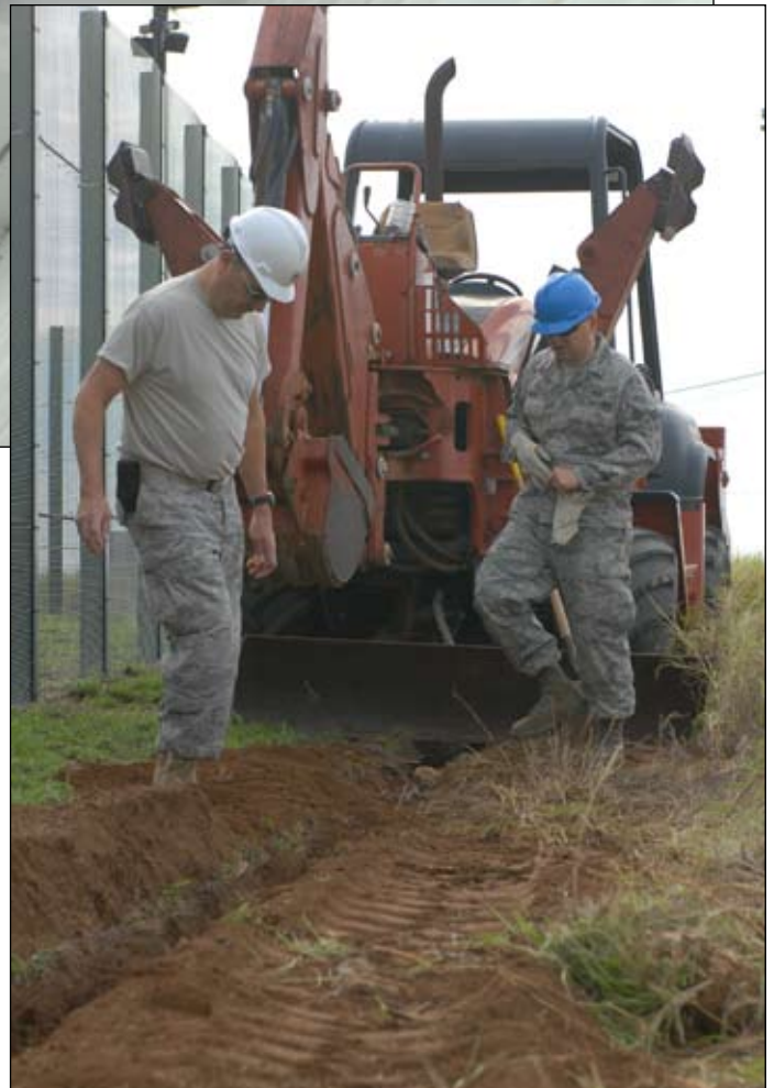
Air Force Master Sgt. Oscar Trevino and Air Force Senior Airman Matthew Lucht with the 190 th Civil Engineering Squadron of the Kansas Air National Guard dig a trench outside of a detention facility, Jan. 7. – JTF Guantanamo photo by Army Spc. Cody Black
