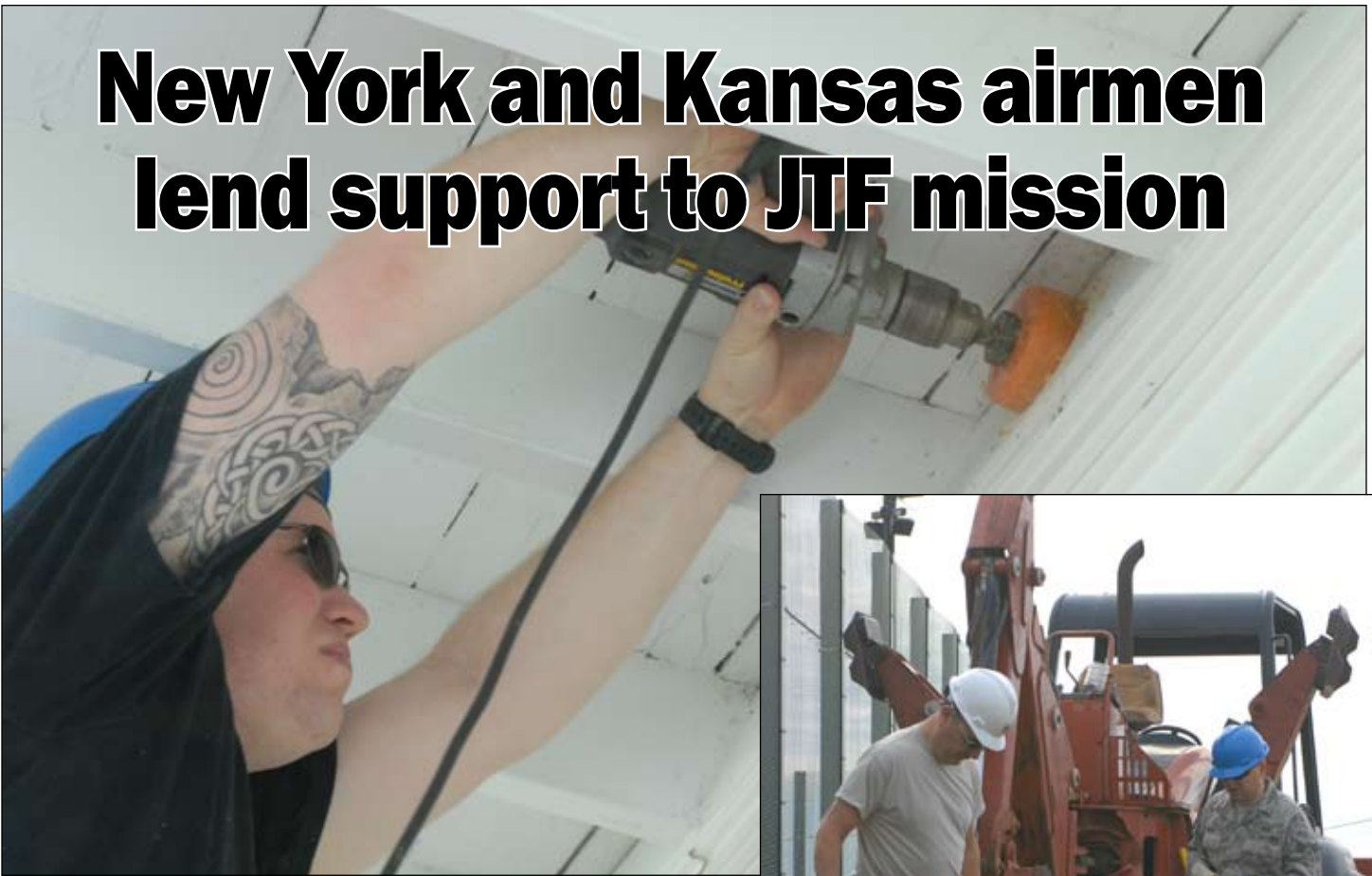
An Airman with the 190 th Civil Engineering Squadron drills into the side of a building while conducting repairs, Jan. 6. – JTF Guantanamo photo by Army Spc. Christopher Vann
