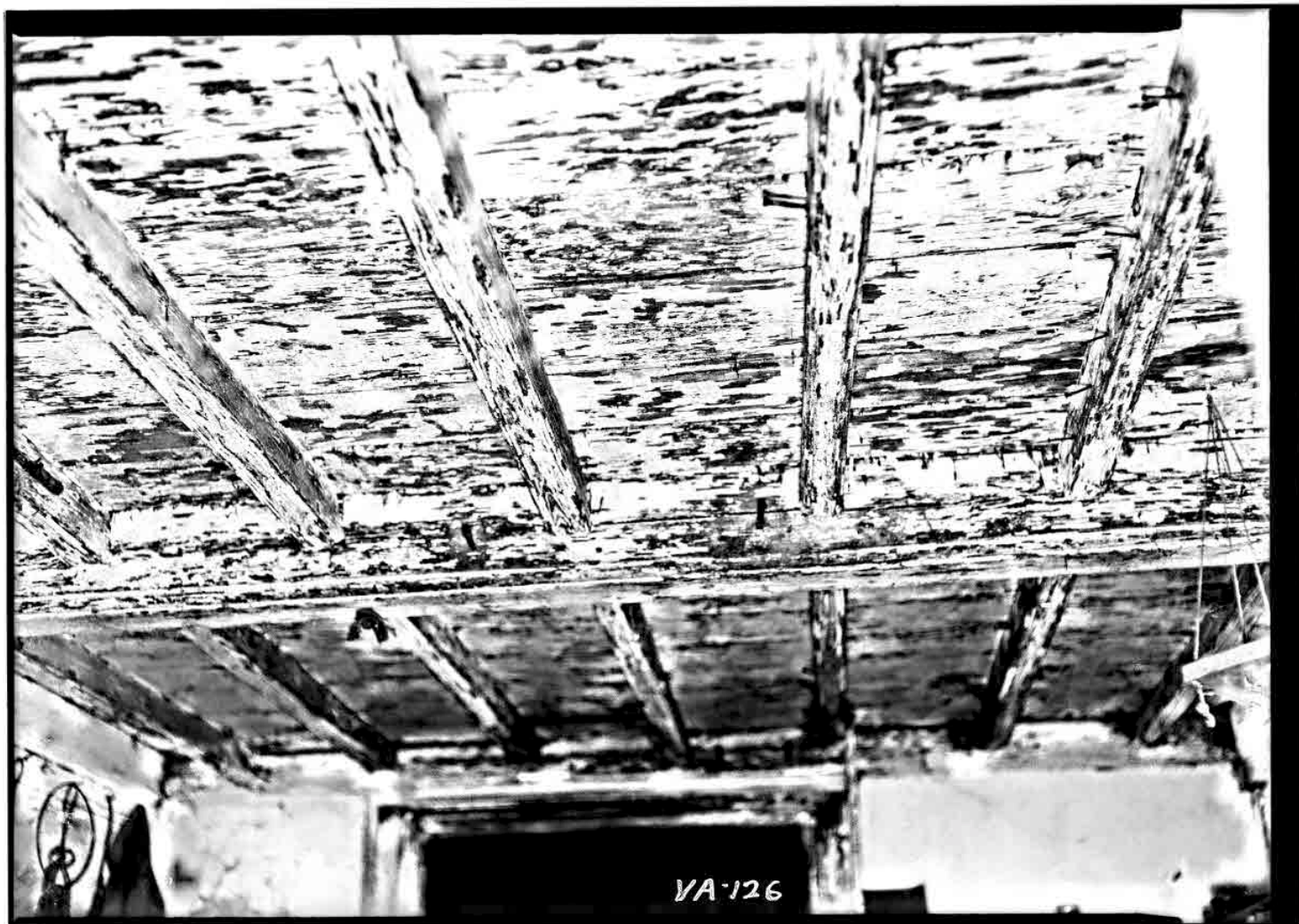
Photo of the Under Side of the Sub-Flooring, for Upstairs, as Seen From the Basement.
